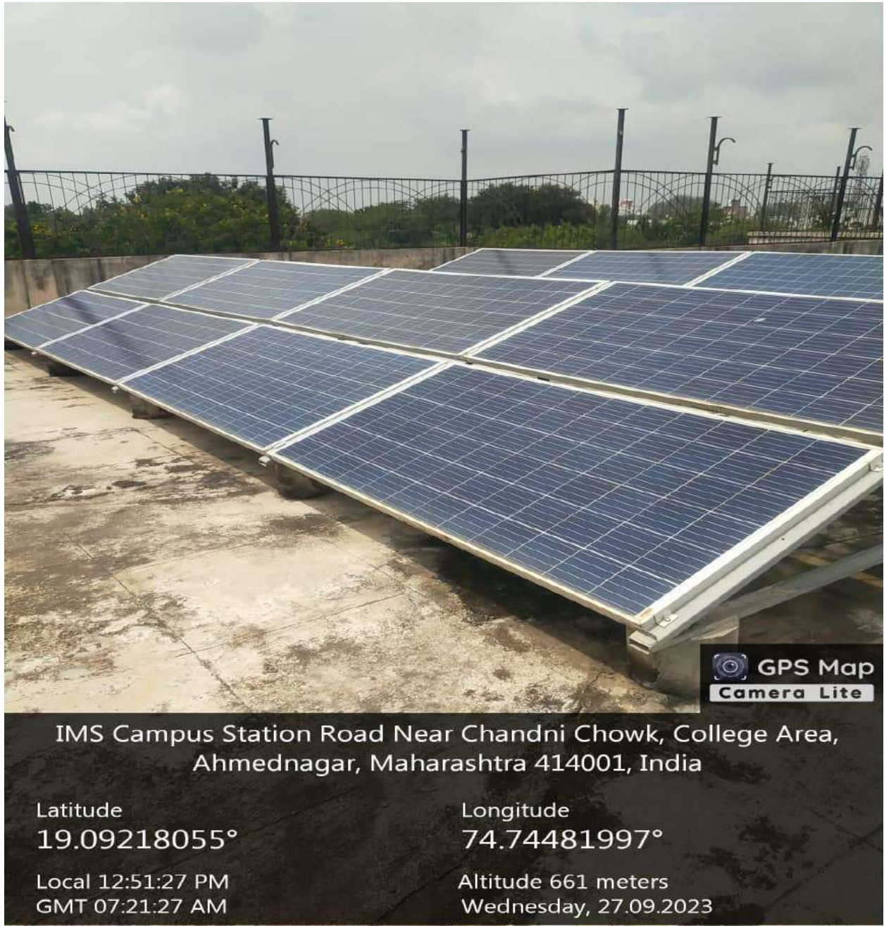
Solar Panel for Electricity Generation (Capacity 10 KW)
